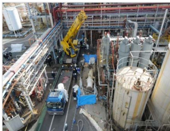
Figure 1.6 polycrystalline silicon manufacturing facility
