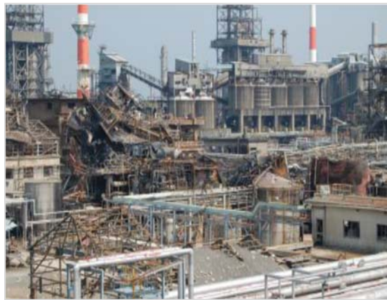
Figure 1.4 Resorcinol production facility
