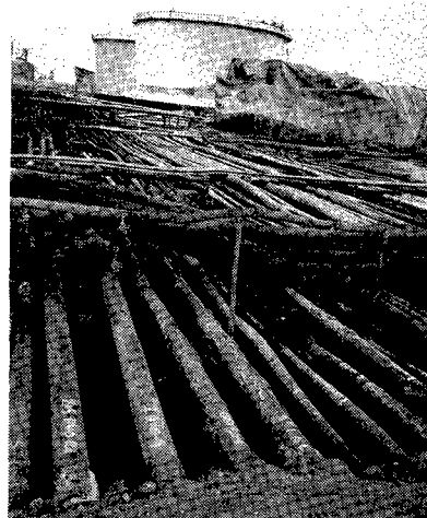
Fig.14 Damaged Pippings by the Tank Fire
