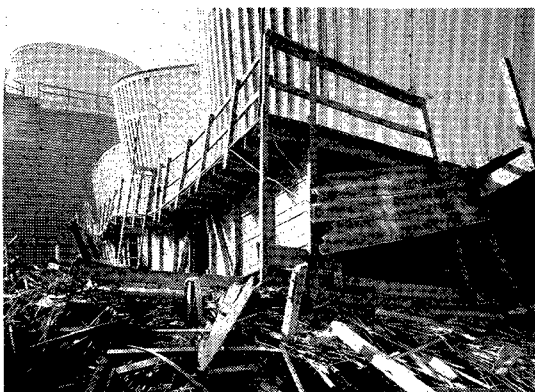
Fig.28 Collapsed Wooden Cooling Tower Structure
