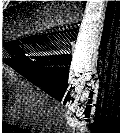
Fig.29 Damaged Support Column of Reinforced Concrete Structure for Colling Towers
