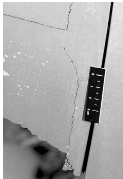
(c) Numerous cracks were also noted in RCC Panel 8.
