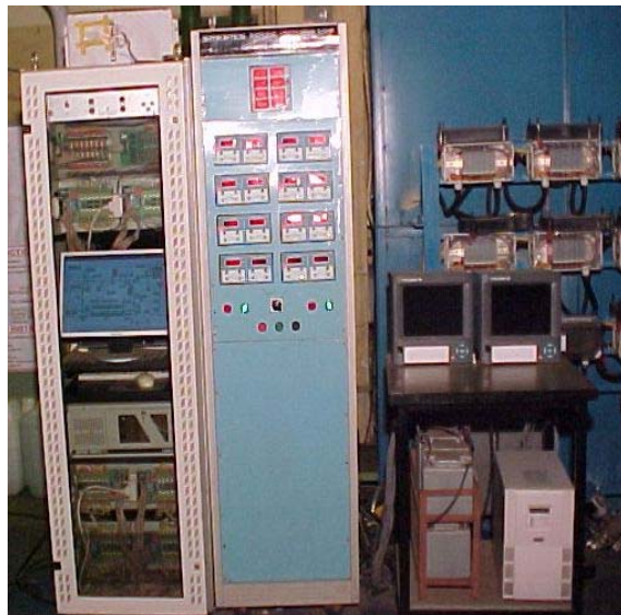
Figure 6-6: Photograph of control panel of SPNCL
