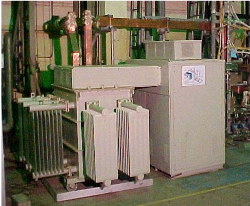
Figure 6-3: Photograph of 200 kW Power supply unit
